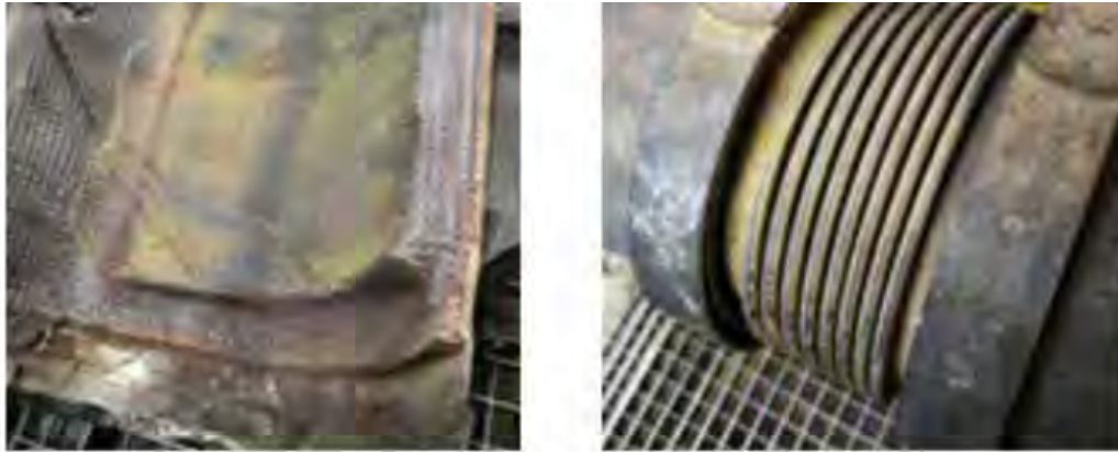
Illustration 1 Exhaust system examples of yellow residual deposits
