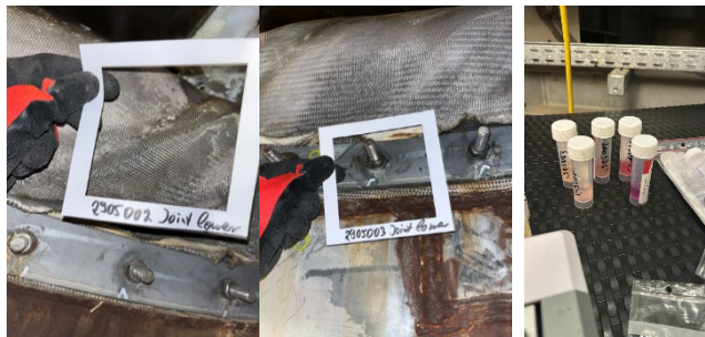
Abb.14&15: Dehnungsfuge Turbine (Expansion Joint)
