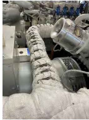
Fig. 66/Fig.67 CHP exhaust pipe insulated calcium-free
