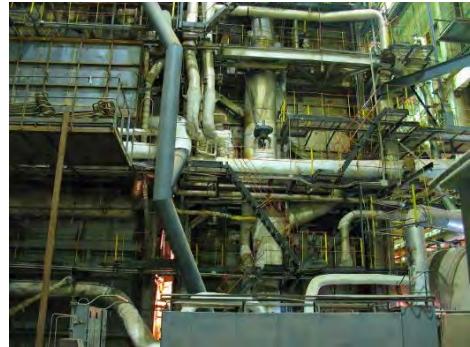
insulation Fig. 8: Power station insulation
