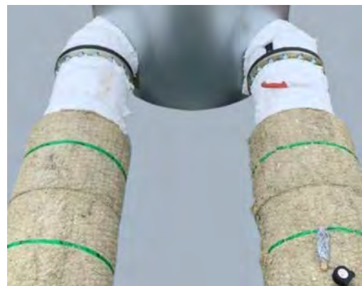
Fig. 81: Industrial insulation with chromate blocker
