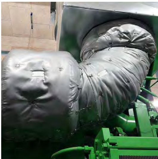
Fig13: Insulating mattresses exhaust area
