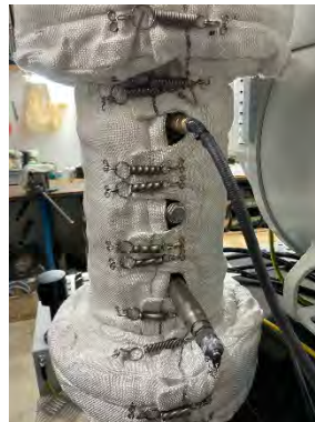
Fig. 68/Fig.69 Exhaust pipe CHP unit insulated calcium-free
